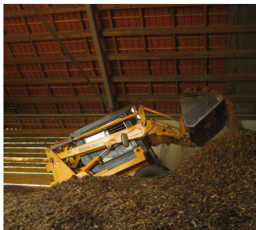
Figure 16: Inside the biomass power plant in Hostětín (photo: Ferenc Kiss)
